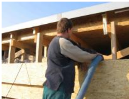
Fig. 1 Passive House A - filling the cavity of the roof with cellulose insulation
