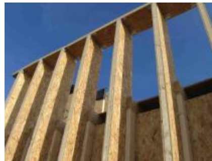
Fig. 2 Passive House B - wood frame structure. The skeleton was made from box-joist members
